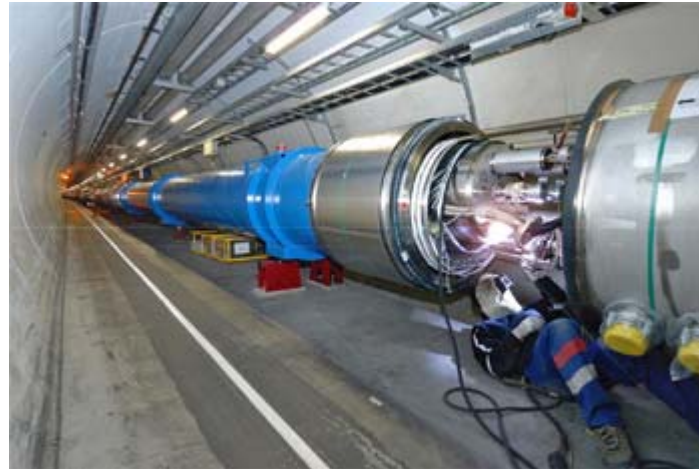
Interconnections on the last sector of the LHC
